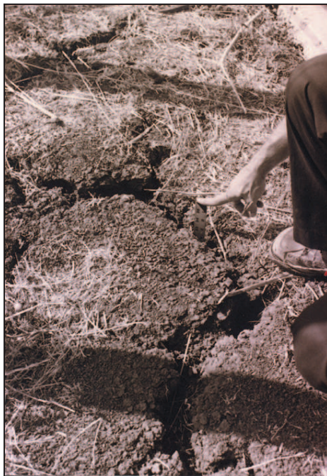
Figure 2: This crack is at least 32 inches deep. The yardstick was easily inserted to this depth; narrower, less straight cracks may extend much deeper.
