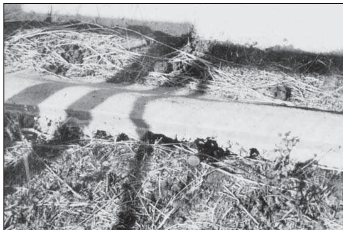
Figure 5: Void created under concrete drainage interceptor ditch by contraction of clay soils.
