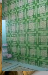
Asbestos backed vinyl in a kitchen.
