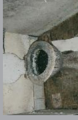
Asbestos cement sheet walls in a toilet.
