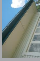
Asbestos cement sheet eaves lining.
